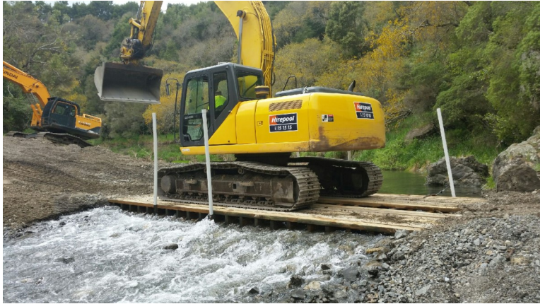
Drift Deck, cheap to build, sits on swampy areas or stream bed
